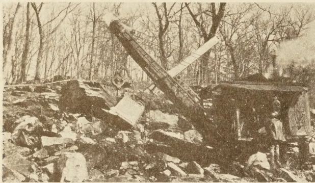
FIGURE 2.—A GOOD SHOVEL PLUS A GOOD OPERATOR CAN HANDLE ROCKS LIKE THIS, BUT THE COST PUTS THIS KIND OF BLASTING INTO A LUXURY CLASS WHICH NO CONTRACTOR CAN ANY LONGER AFFORD
